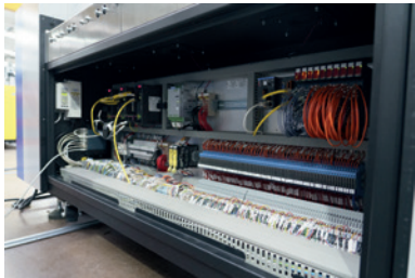
CE and UL certified electrical installation.
